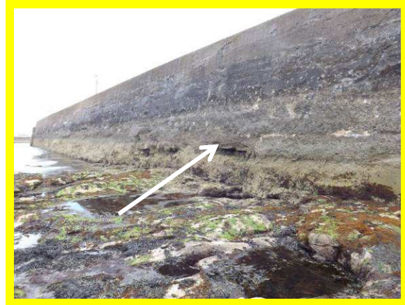
Increased depth of abrasion hole 1701/C07 2016
