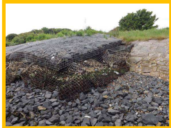
Undermining due to failure of lower baskets at northern end.
