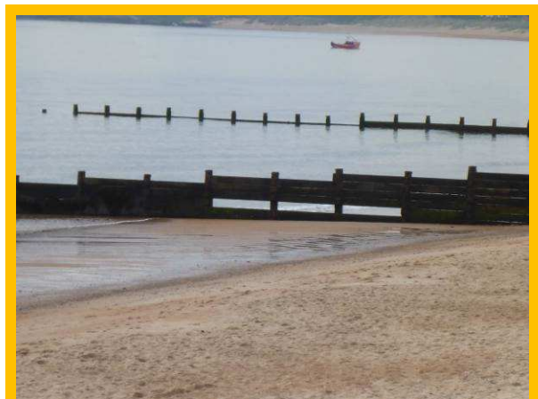
Missing timber planks on groynes (/4201C07)
