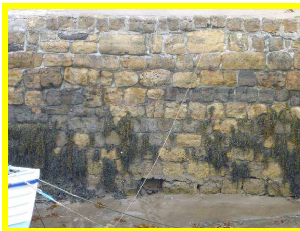
Missing block at toe of Beadnell Harbour wall (inner face of northern wall) (/1701C52)
