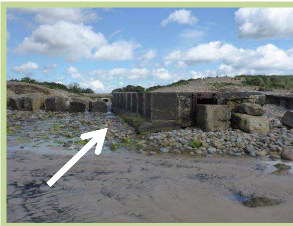
Drainage occurring alongside of remnant outfall structure through gravel, cobbles and boulders (/3201C09)
