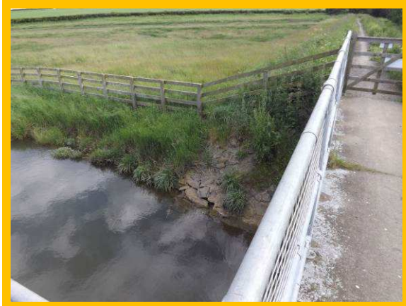
1401/C01 – undermining of edge protection.
