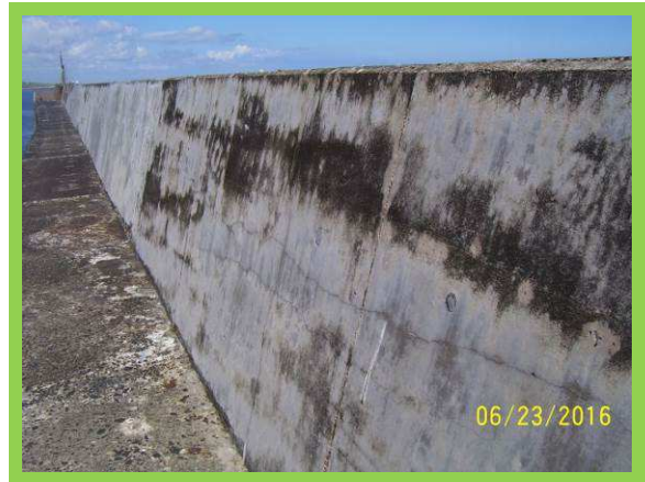
1701/C21 Good condition, some cracks in original deck but no significant damage
