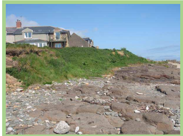
Inactive slopes with rock ledge at toe, with one minor area of slippage (/2201C14)
