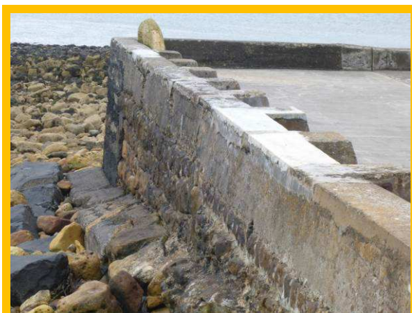
Abrasion and undermining of Beadnell Harbour wall (outer face of eastern wall) (/1701C47)
