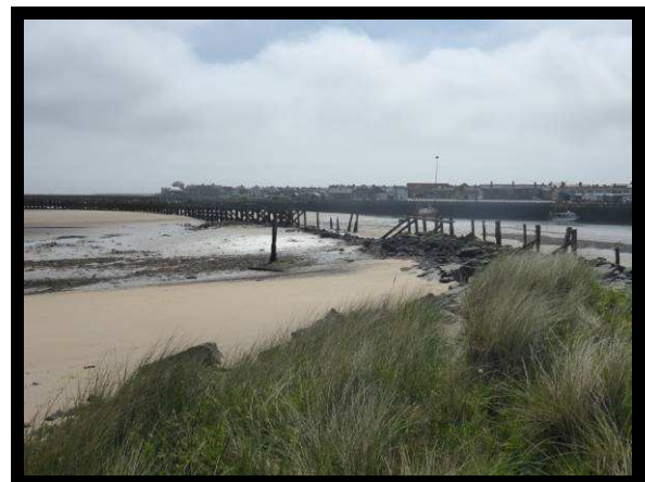
Dilapidated North Jetty (no asset reference)
