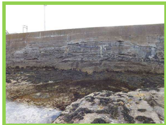
Old crack not noticeably worse 1701/C07
