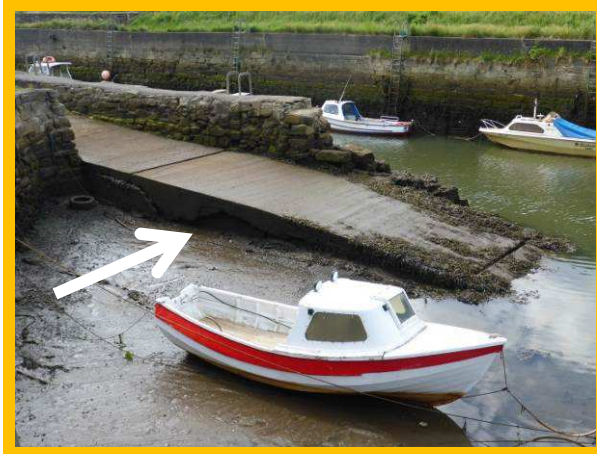
Undermining at toe on inner face of boat ramp (/4401C05)
