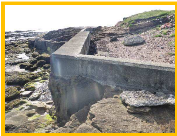
Seawall with undermining and outflanking (/3501C08)
