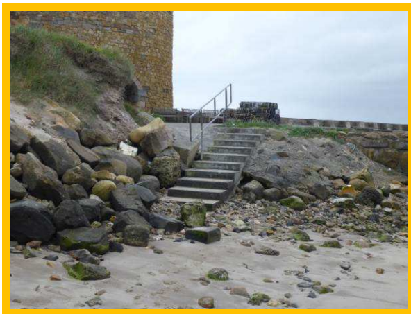
Missing block at toe of Beadnell Harbour wall (inner face of northern wall) (/1701C53)
