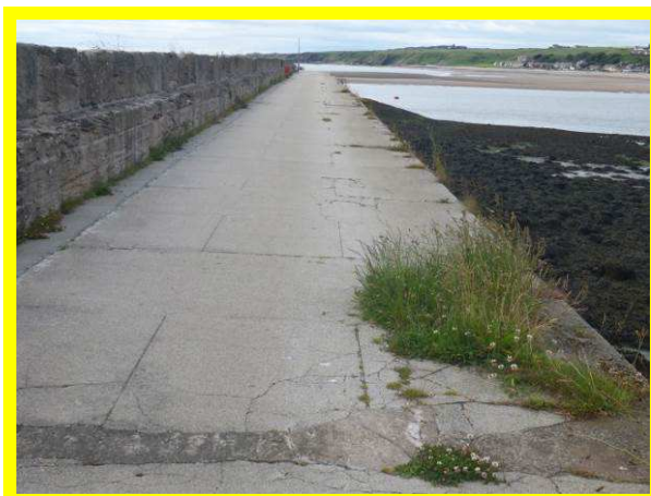
Older (inland) sections of cracked deck and abraded wave wall on Berwick Pier (/0701C14)
