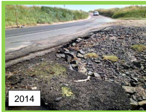
Localised erosion damage to road at Chare Ends in 2014 (4901c01)
