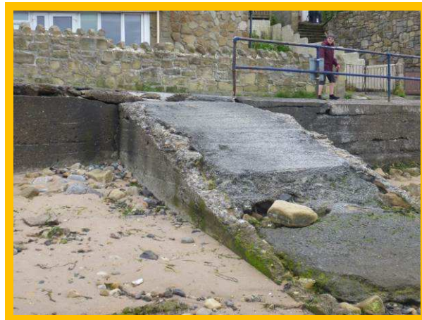
Access ramp to Little Shore Wave Basin in poor condition (/3001C10)
