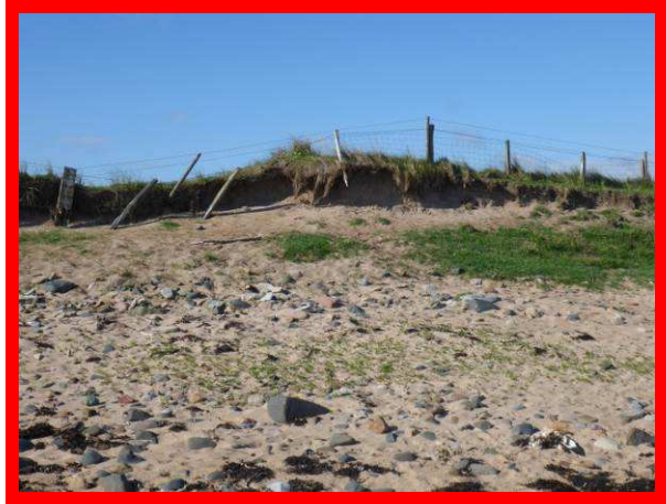
Local erosion affecting fence line (/2501C01)
