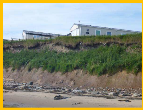
Active slumping at northern section fronting caravan park (/3501C05)
