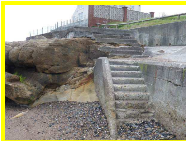
Heavily abraded access steps to foreshore (/3101C02)
