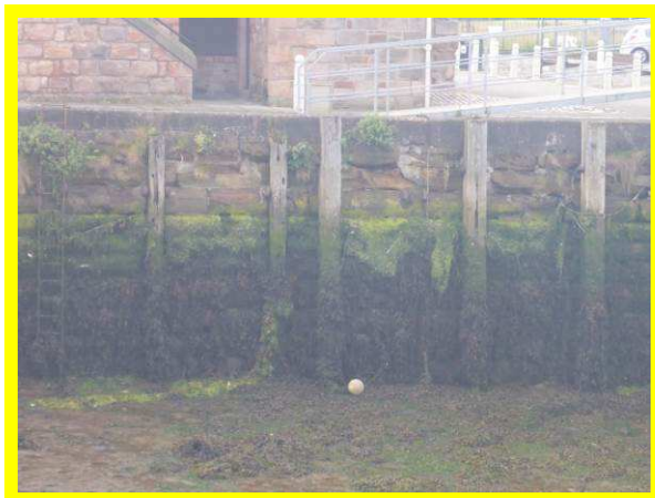
Masonry quay walls in dock area in fair overall condition with some open joints, cracks and abrasion (/0801C03)
