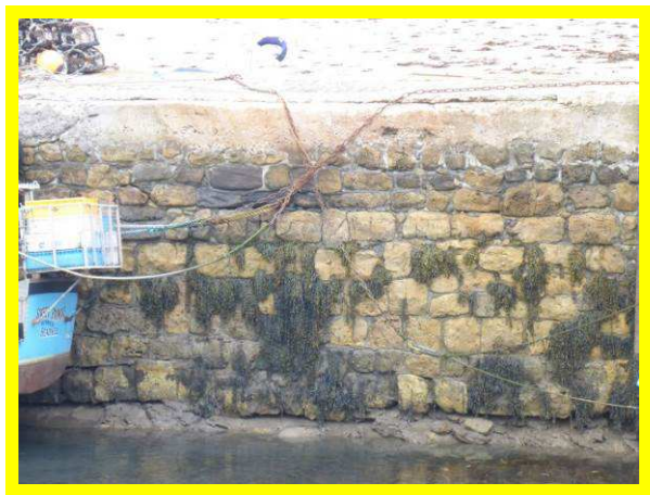
Undermining of Beadnell Harbour wall (inner face of northern wall) (/1701C51)
