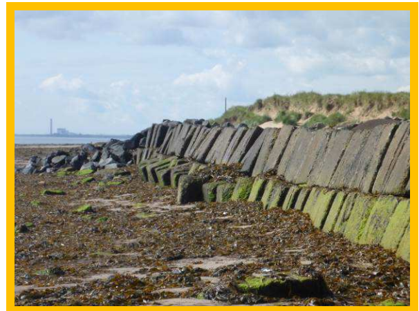
Rotational displacement at southern end of concrete block revetment (/3201C04)
