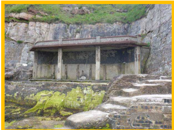
Concrete pavilion structure in fair/poor condition (/0701C02)
