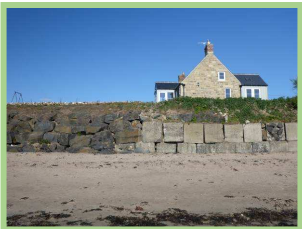
Stacked concrete blocks (original scheme) and rock revetment (emergency scheme) at northern end of Boulmer village (/2601C02)
