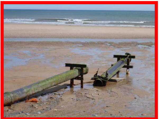
Collapsed section of outfall pipe in southern end of Druridge Bay (/3201C16)
