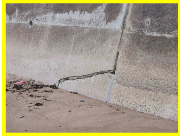
1001 c03 – Crack noted previously 2008 through to 2014.
