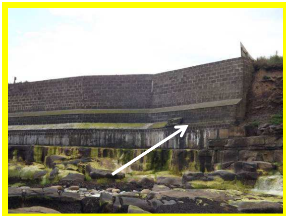
Damage of lower coping 1701/C02 - 2016
