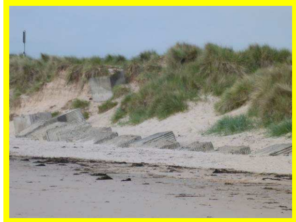
Minor slumping in dunes protected by concrete blocks by Alnmouth Golf Clubhouse (/2701C08)
