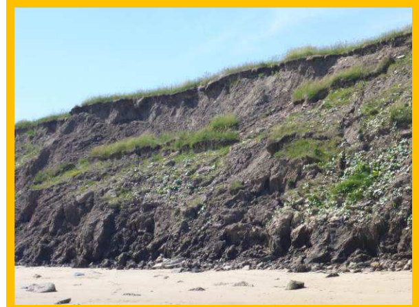
Eroding cliffs south of Cambois House (/3901C01)
