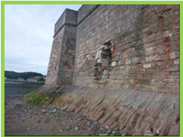
Abrasion to toe apron where present (/0801C06)
