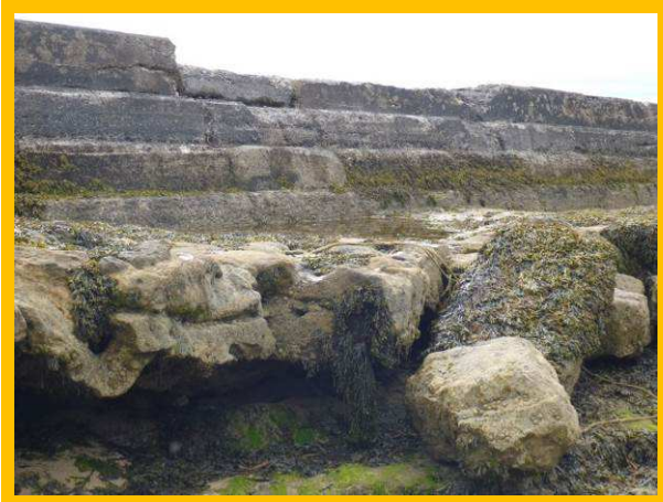
Abrasion, damage and rock undercutting along the breakwater (/0701C04)
