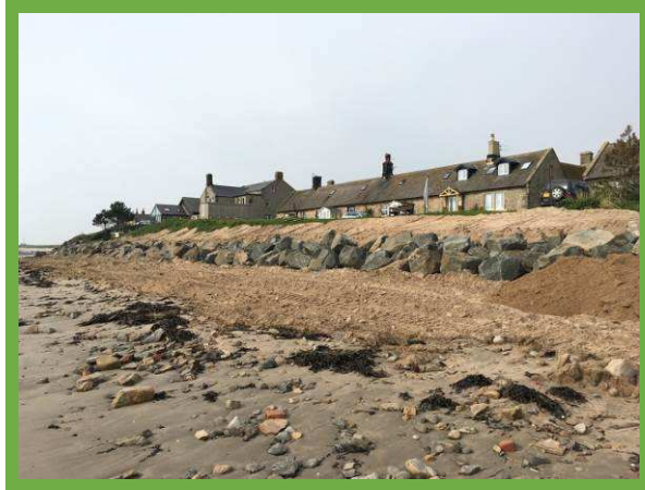
New rock revetment toe to protect previous central 'gap' at Boulmer village (/2601C03) – constructed May 2016
