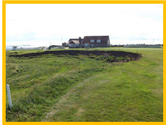
1501/C07 – significant slip at crest of slope
