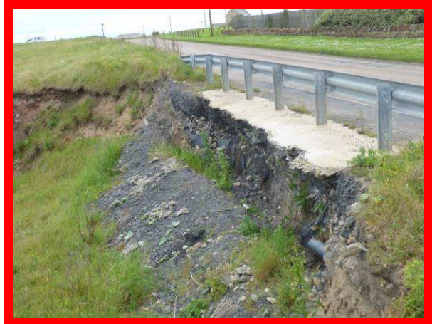
Failed section of cliff adjacent to coast road (/3201C22)
