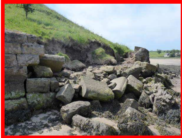
Collapsed section of wall at Church Hill (/2801C13)
