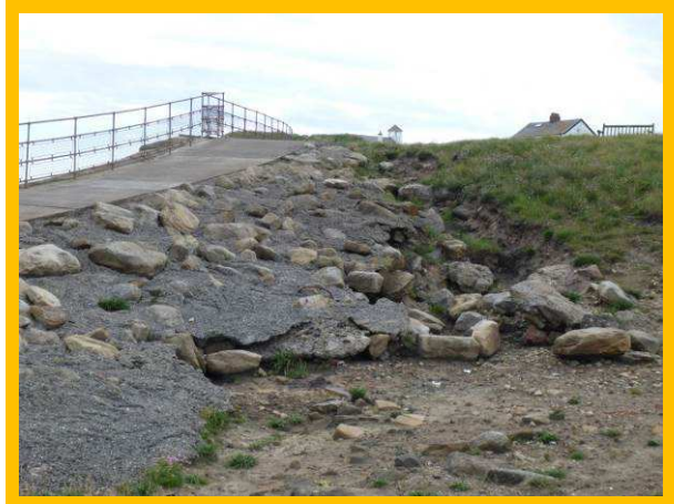
Break-up of poured concrete slurry and erosion of slope (/4401C11)
