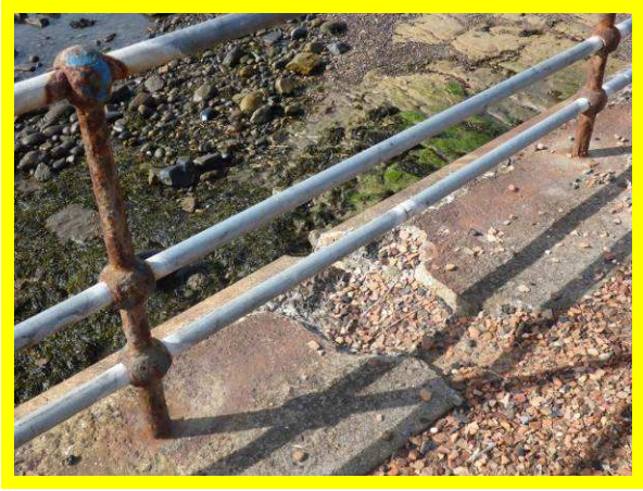
Local crest damage to Church Point seawall (/3601C12)
