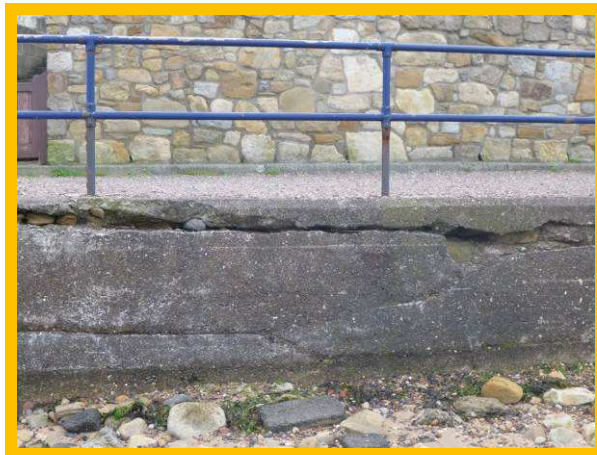
Sea wall along Bay View in poor overall condition (/3001C10)
