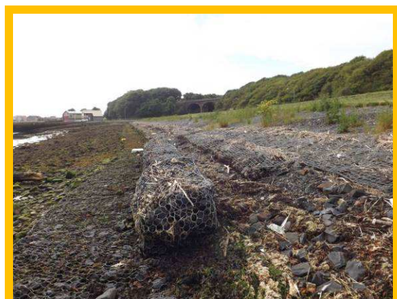
Deterioration due to corrosion of wrapped basket 2016, 901c04.
