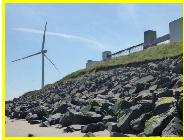
Composite defence with corroded steel breastwork (/4001C02)
