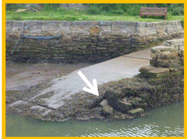
Collapsed wall on outer face of boat ramp (/4401C05)
