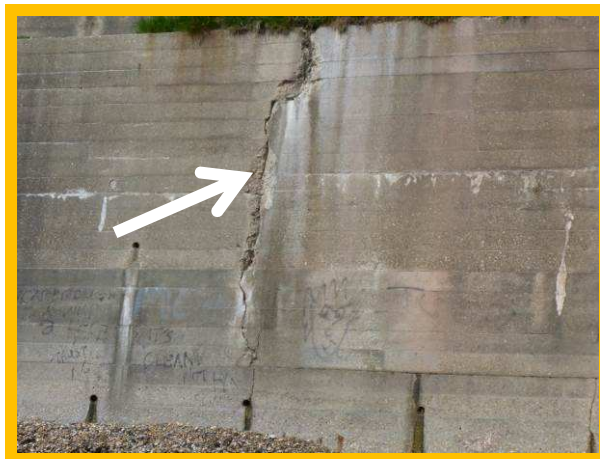
One of three notable vertical cracks in the sea wall (/4401C17)
