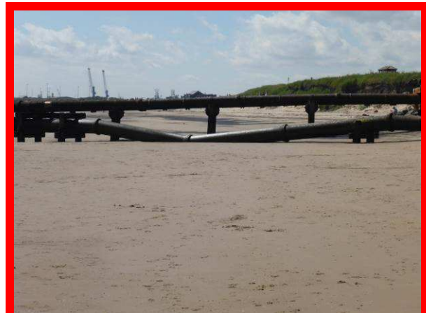
Failed section of outfall pipe (/3901C05)
