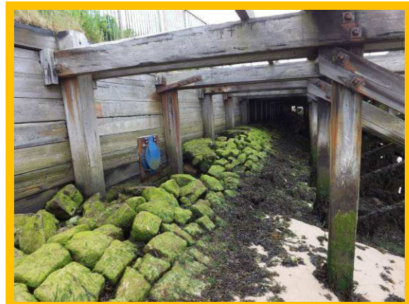
901c07 – further displacement of revetment, associated with maintenance of flap valve.
