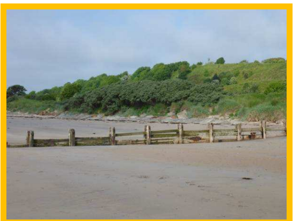
Missing timber planks on fifth (southerly) groyne in field of five groynes (/2701C05)
