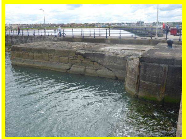
Poor condition at junction of South Pier and South Jetty (seaward face) (/3101C01)
