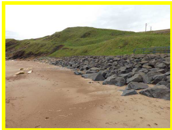
1001 c04/ 05 – higher beach levels, vegetation to previous coastal slope slippage..
