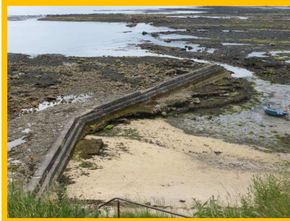
Green's Haven Breakwater remains in poor condition but still retains beach sand (/0701C04)
