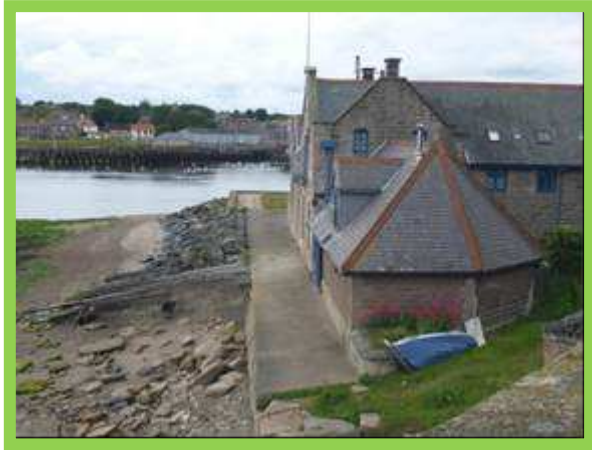
Rock revetment in good overall condition with wall in fair overall condition (/0801C05 & C04)
