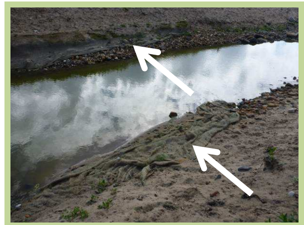
Exposure of geotextile on re-graded side slopes of newly 'daylighted' open channel section (/3201C09)
