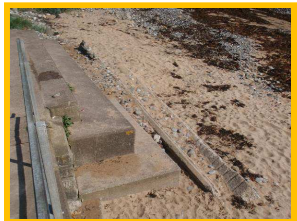
Detached toe beam at northern bridge abutment (/2501C01)
