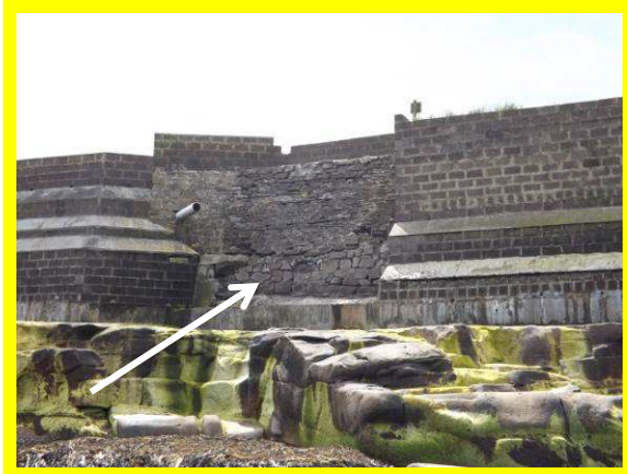
1701/C03 2016, requires repointing.
