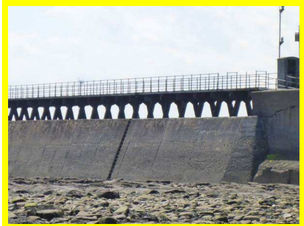
Generally fair condition of main Blyth East Pier substructure (although superstructure in poorer condition) (/4001C05)
