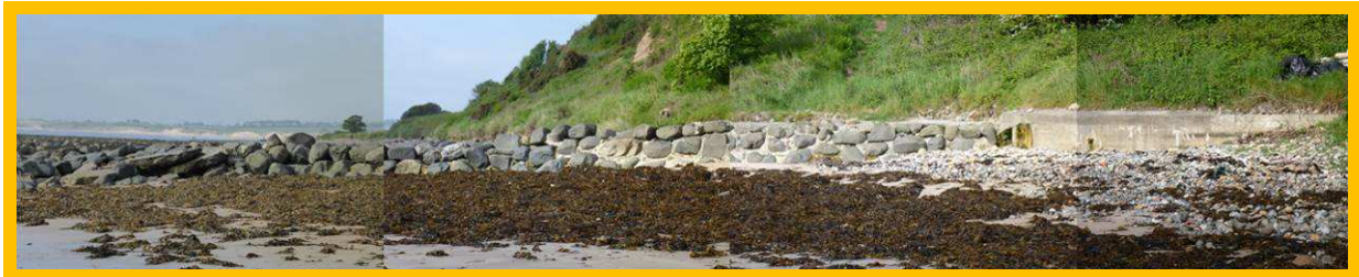
Breakwater wall at Marden Rocks headland in fair to poor condition (/2701C03)
