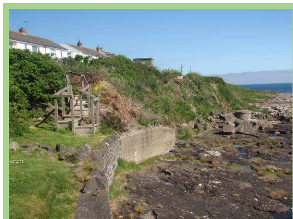
Stable slopes and masonry wall north of Craster Harbour north pier (/2201C02)
