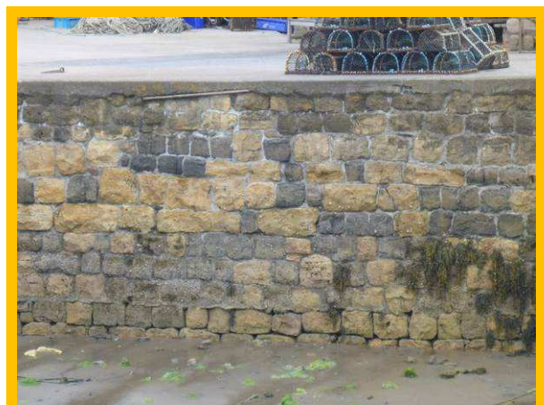
Open joints between blocks on Beadnell Harbour wall (inner face of eastern wall) (/1701C51)
