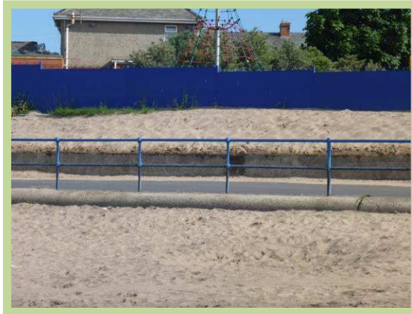
High beach levels and wind-blown sand to rear of promenade in northern sections of Newbiggin Bay (/3601C06)
