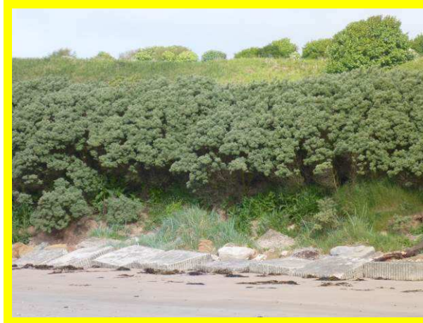
Relatively stable dunes protected by concrete blocks in north of Alnmouth Bay (/2701C06)
