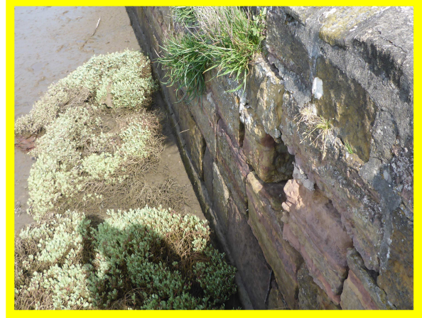
Missing block in masonry wall (/2801C06)
