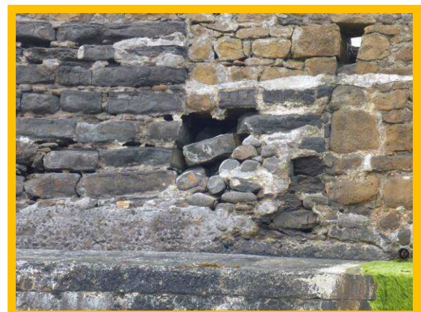
Voiding within seawall at Beadnell North (Nacker's Hole) (/1701C36)
