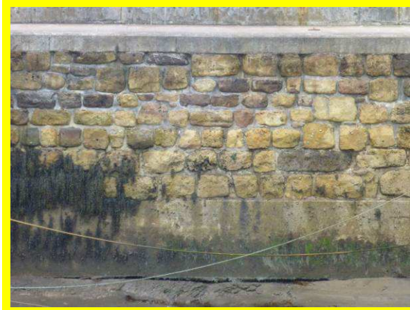
Undermining of Beadnell Harbour wall (inner face of southern wall) (/1701C51)
