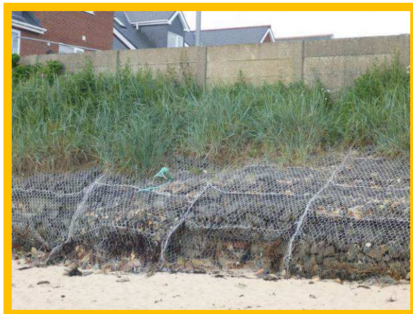
Failing gabions protecting very narrow strip of dunes (/4201C03)
