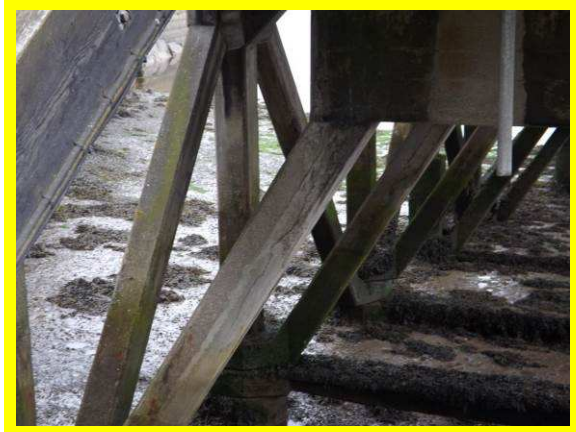
901c07 – evidence of concrete spalling to support structure of RNLI building.
