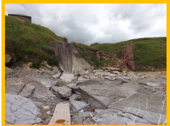
1101/c04 Outfall and concrete slope protection, cracked and weeping water.
