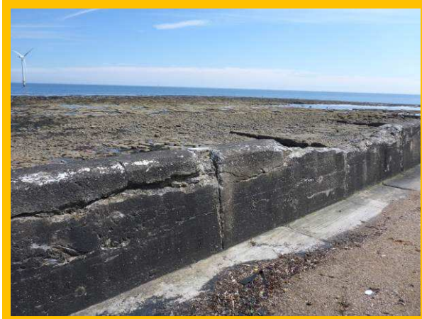
Damaged crest wall and deck of landward section of Blyth East Pier (/4001C04)
