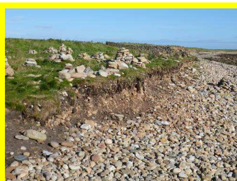
Erosion and undermining of grassed shingle on north side of ness (4901c14).
