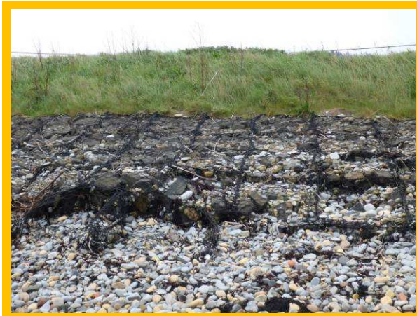
Failing mattresses at Beadnell North (Lady's Hole) (/1701C40)
