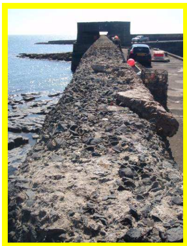
Abrasion and spalling on crest wall of north pier (/2201C03)
