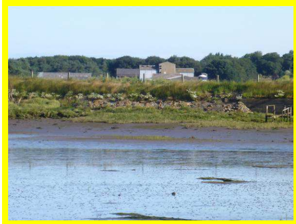
1401C14 – Fair condition revetted bank, but local maintenance would be beneficial
