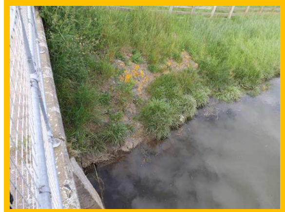
1401/ C01, undermining of edge protection. .
