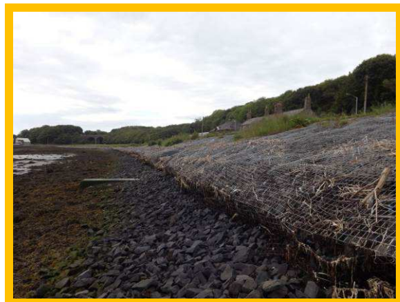
Loss of toe and local damage at outfall 2016, 901c04.
