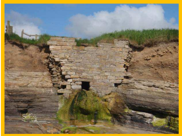
Poor condition retaining wall (/2501C01)
