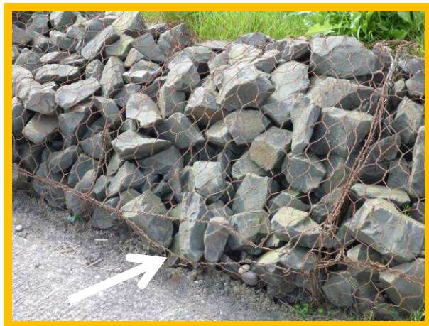
Break-up of gabion baskets (/4401C19)
