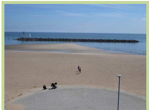
Detached breakwater in central Newbiggin Bay remains in very good condition with salient/tombolo developed in lee (/3601C13)
