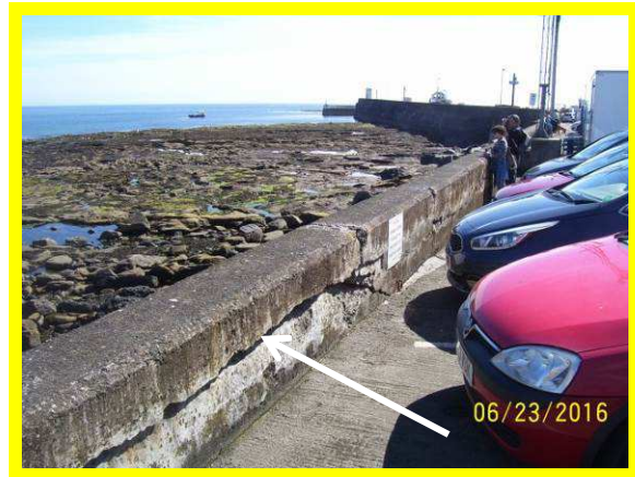
Old crack not noticeably worse 1701/C06
