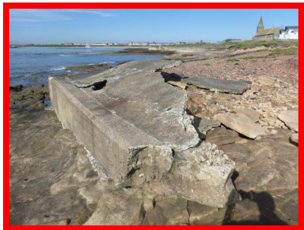
Seawall actively breaking-up since at least 2008 (/3501C10)
