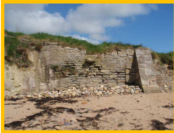
Poor condition retaining wall (/2501C01)
