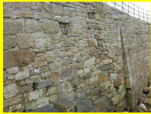
Missing mortar and gaps between blocks (/4401C11)
