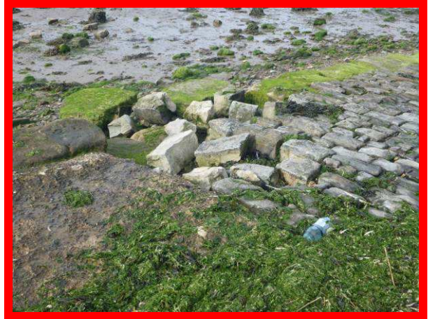
Local failed section of slipway over foreshore outfall (/0801C07)
