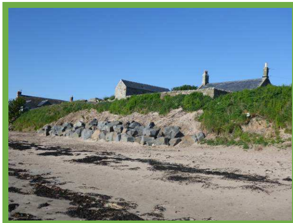
New rock revetment toe to locally protect isolated property at northern end of Boulmer village (/2601C01) – constructed May 2016
