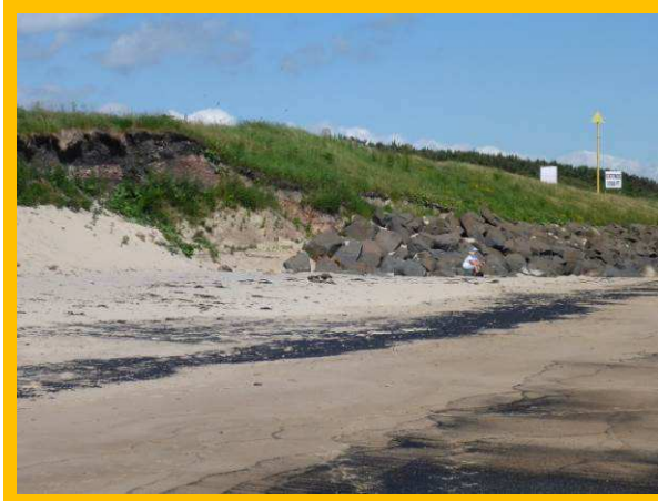
Erosion of cliffs at terminal end of rock revetment (/3901C03)
