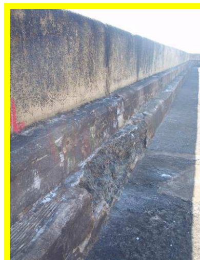
Abrasion and spalling on inner face toe of crest wall of south pier (/2201C11)
